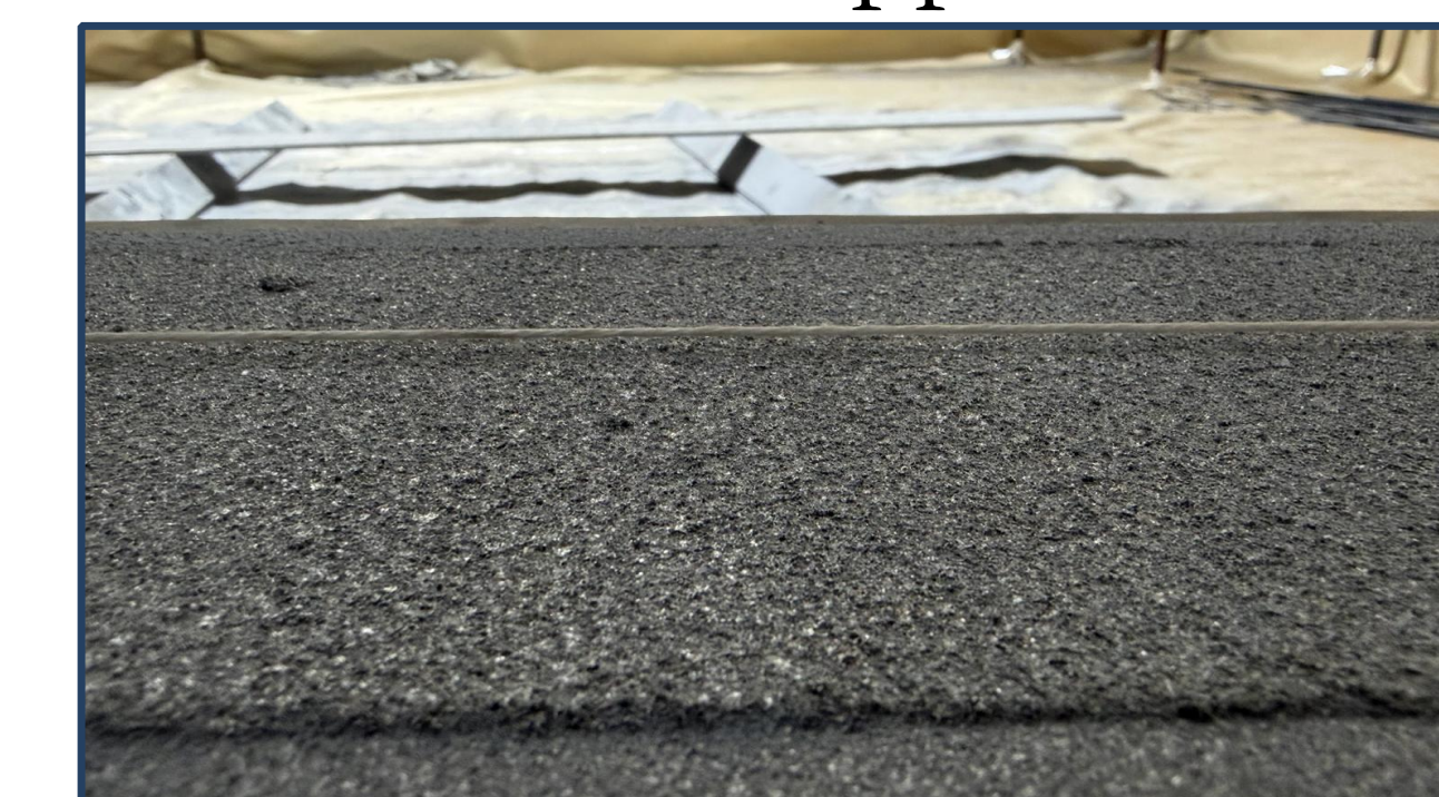
Control plate with TSN, string demonstrates deflection ( >1/8'' )
